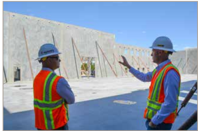
City Administrator Jason Walker and Power Director Joel Eves discuss the construction of the new power facility and generation plant.
