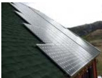
Monocrystalline solar panels.
