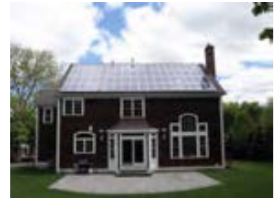
Roof-mounted solar array for large power capacity.
