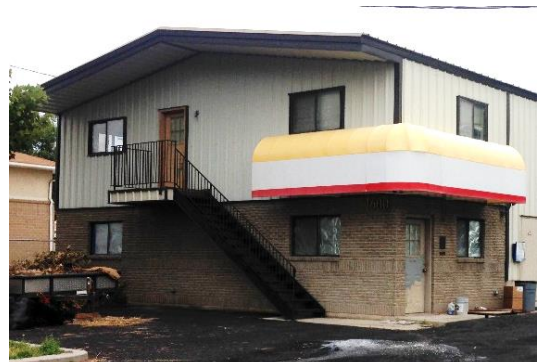
Figure 85 – Metal used is an industrial grade and has the appearance of standing seam metal which detracts from the architectural quality of the building.
