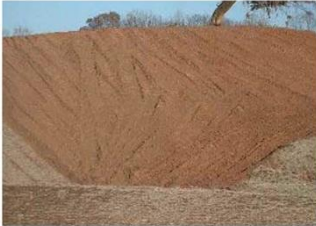
Soils exposed from land grading activities are very vulnerable to erosion
